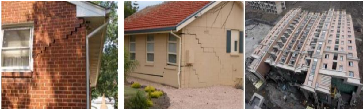
(a) Failure of wall and façade (b) Failure of wall and windows (c) Failure of a building (Song, 2010)
